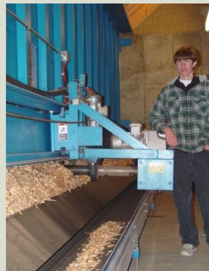
Biomass Heating System in Darby, MT will save the community $100,000+ during the '07-'08 heating season.
